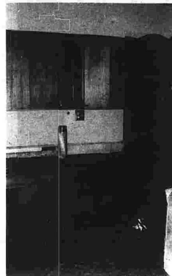
Installation of new kitchen cabinets was included in the process in the interior of the house.
